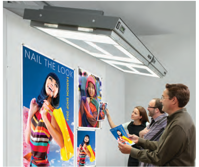
Bracket mounted GLE-1032PH luminaires with Munsell N8/ neutral gray wall panels
